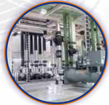
Machine Room Golden Tulip Lucknow
